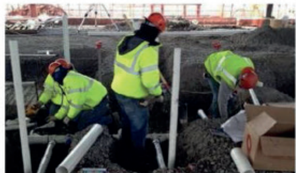
CHW, Plumbing, Fire Fighting, Condensate Drain, MVEAD, ACRAD Works for LELABO & TROMBORG, Al Shaya Group
