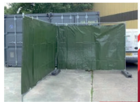
Heras Fencing With Netting
